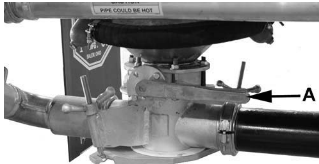
Figure 5-6 – Discharge Valve Closed
