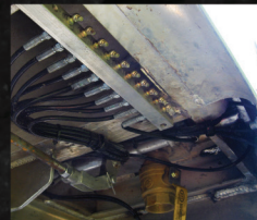
Central Grease Block and Floor Drain Valve
